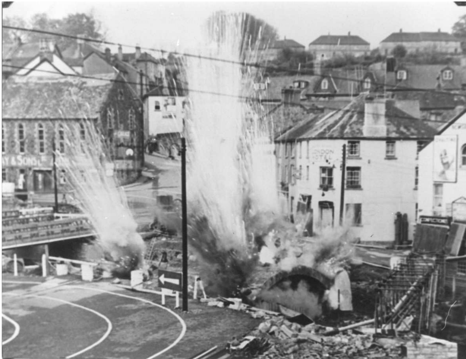
Document 5 – Blowing up West Bridge, 1957.
